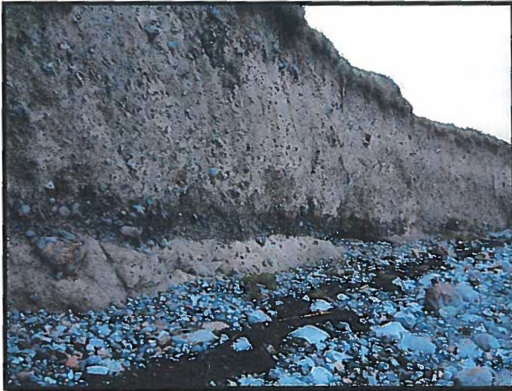
Another view of eroding cliff face from foreshore
